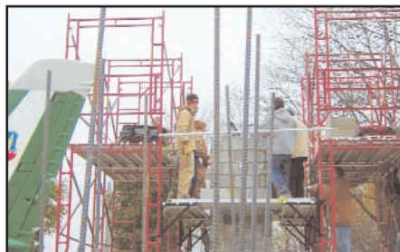
The team works to construct the four towers that will serve as a base for a canopy that will enclose a F56 Saber jet used during the Vietnam War.
